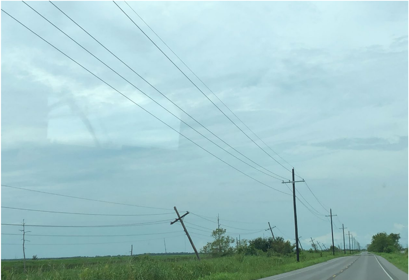
New poles and old poles Dulac, Terrebonne Parish
