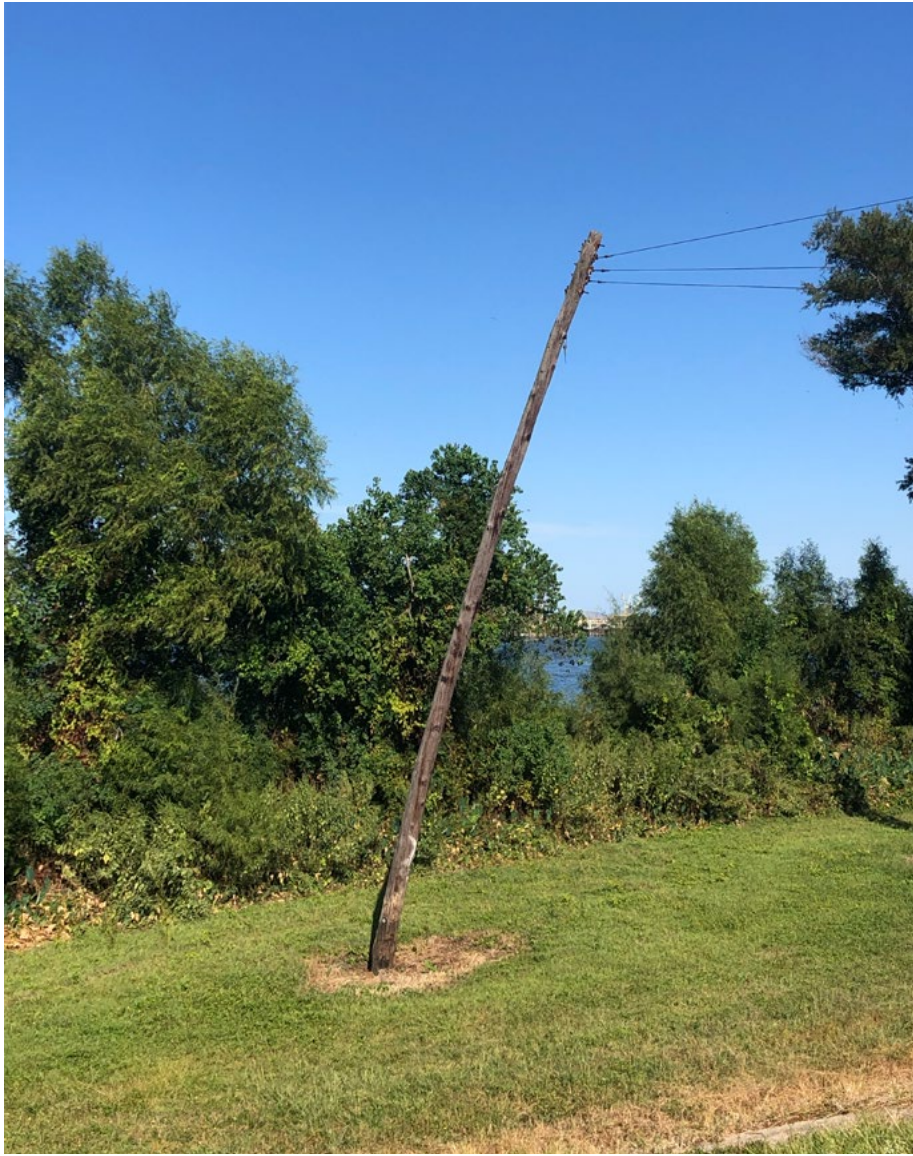
Leaning pole on the levee Algiers, New Orleans
